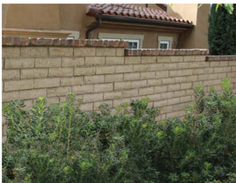
Slumped Block with Brick Cap
